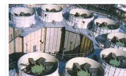
Cooling Tower / Air Fin Cooler
